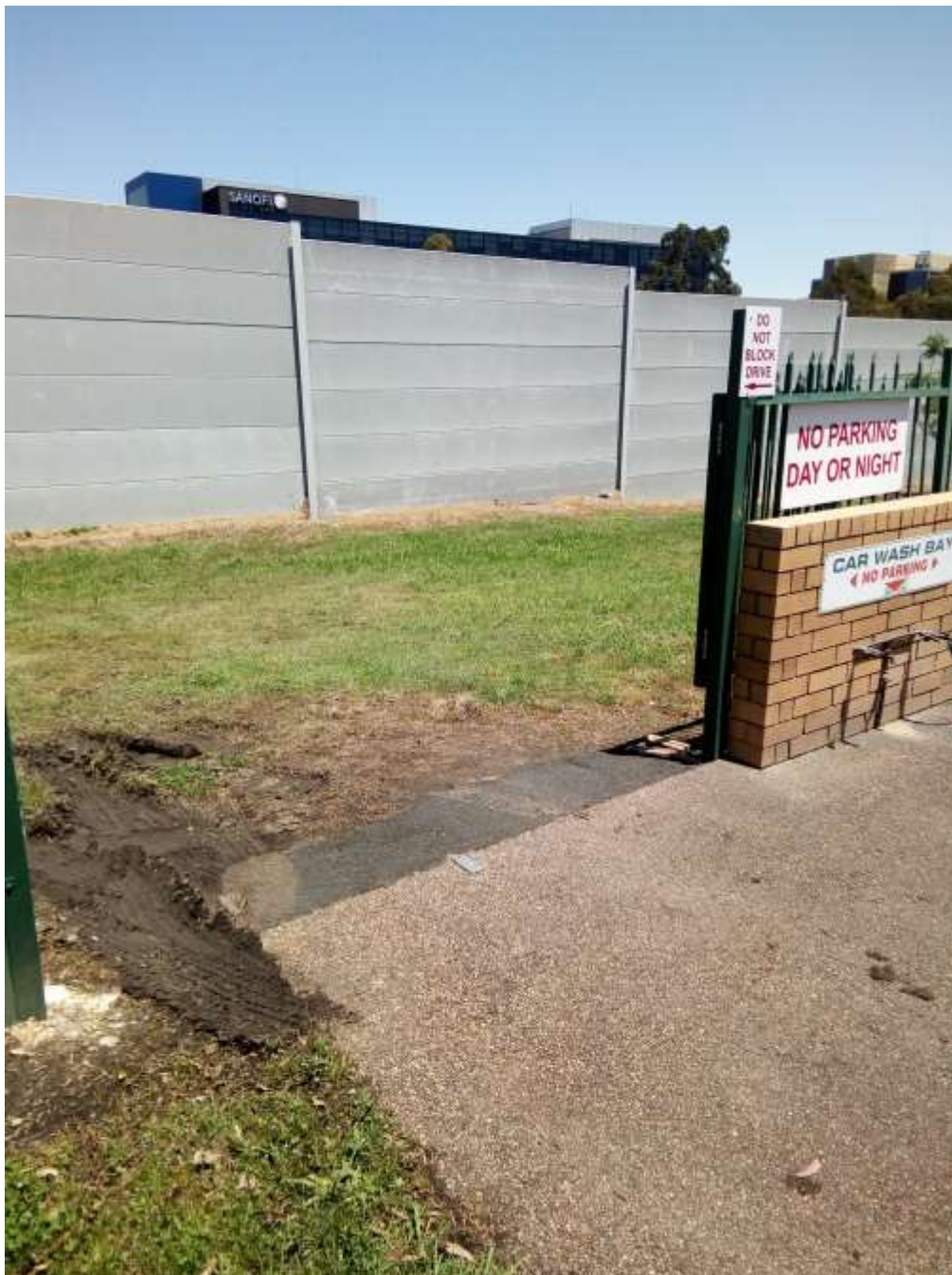
Damaged grass and soil on council land due to car parking on 20 th of November 2018
