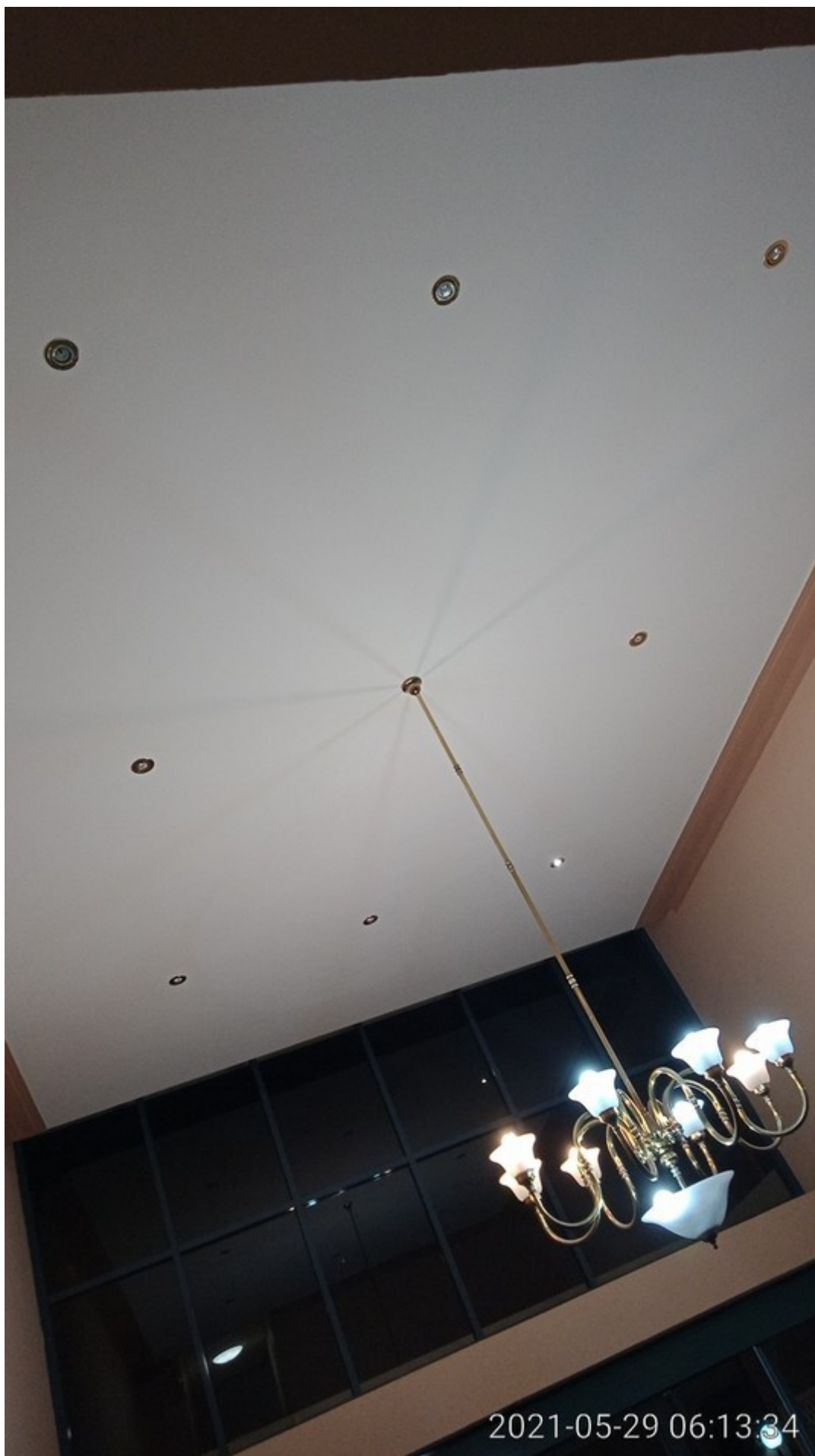
b) Block B, none of eight down-lights operational
