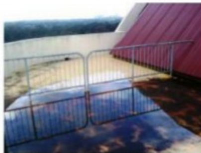
Standing water to flat roof deck, Block B
