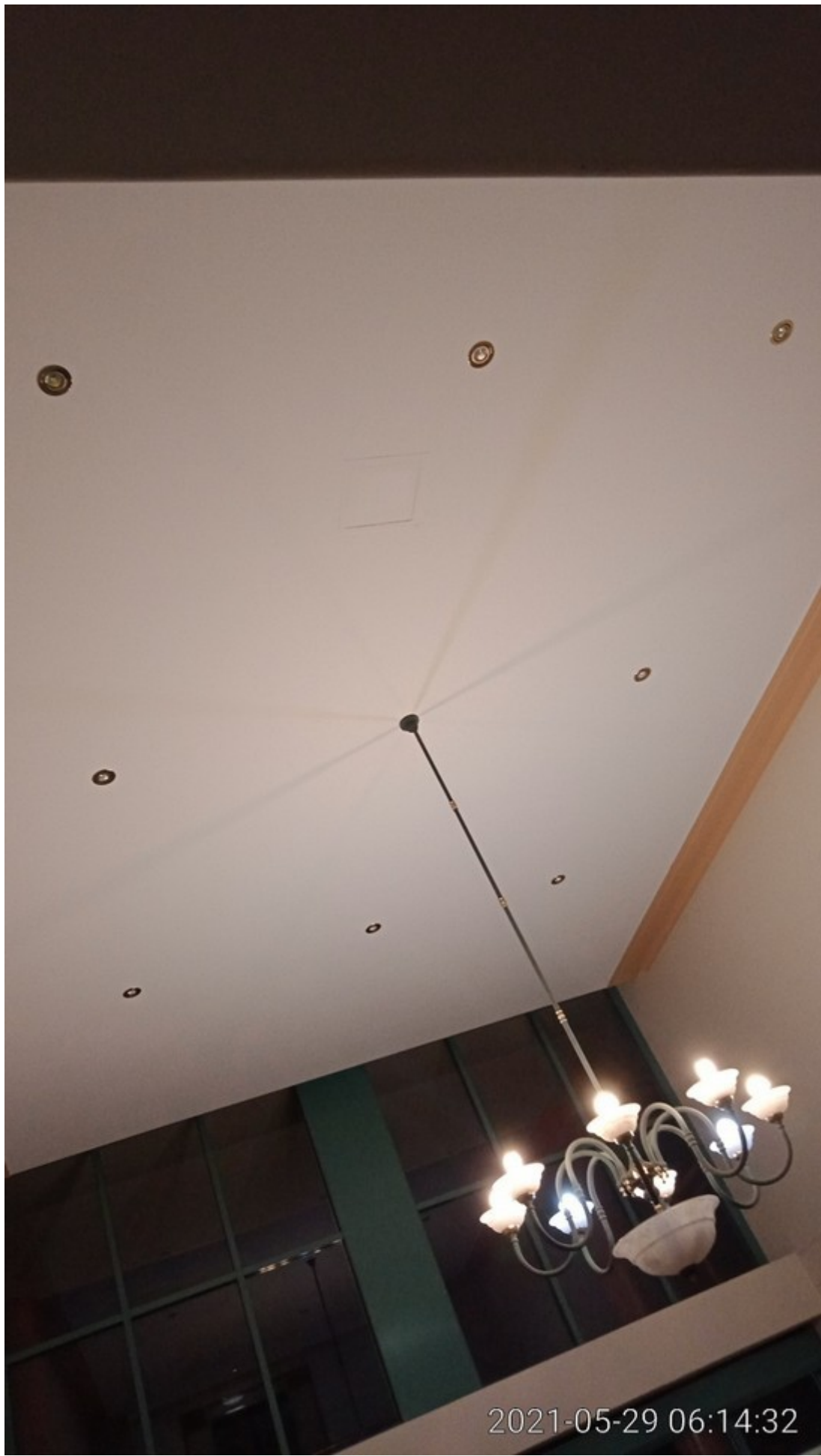
c) Block C, none of eight down-lights operational
