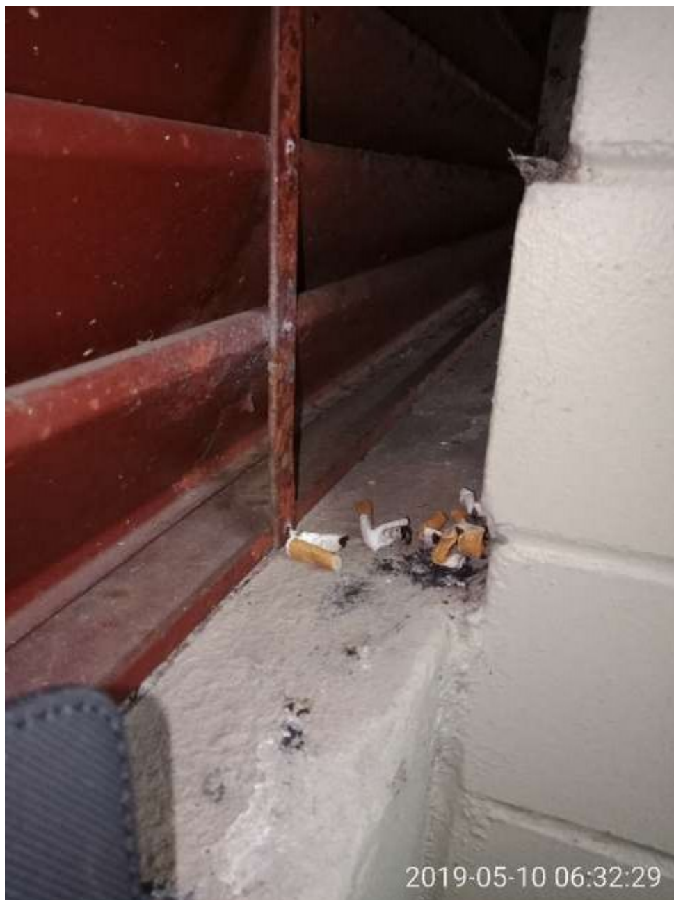
Example of hiding cigarette butts near louvres behind fire door 2 below Block A in May 2019:
