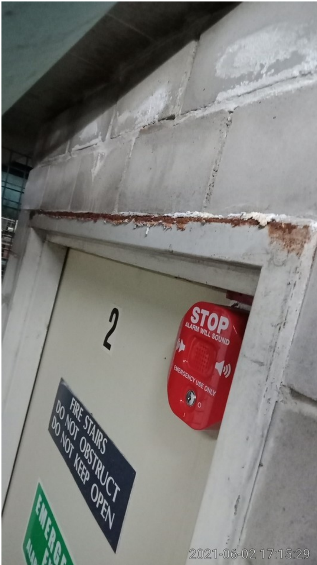
25 Rusted frame of fire door for six years – Block A basement
