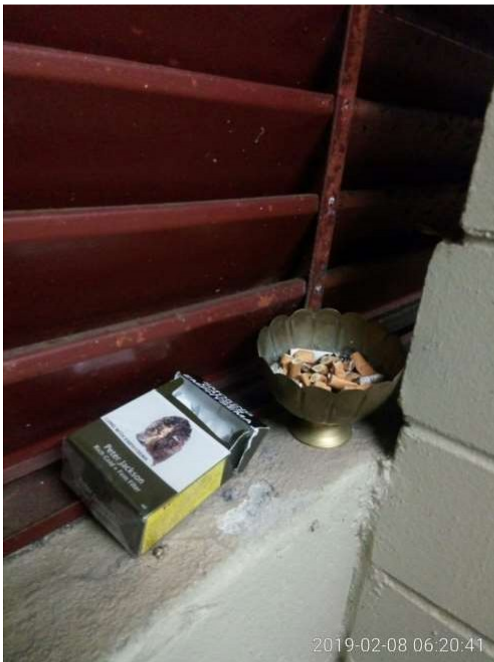
Example of hiding cigarette butts near louvres behind fire door 2 below Block A in February 2019:
