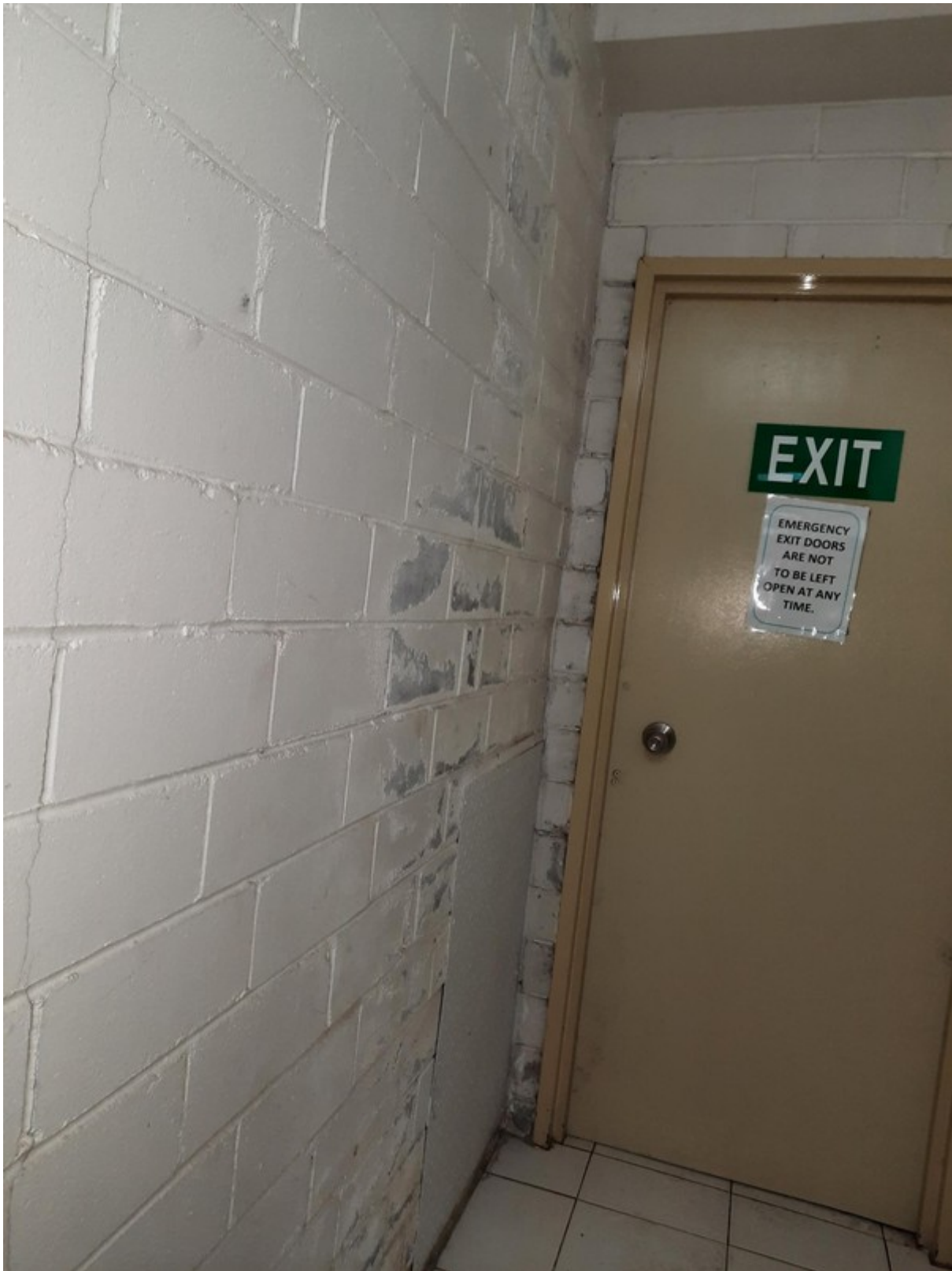
Wall was repainted in July 2021, but the metal plate stayed as is on 1 st of October 2021.
