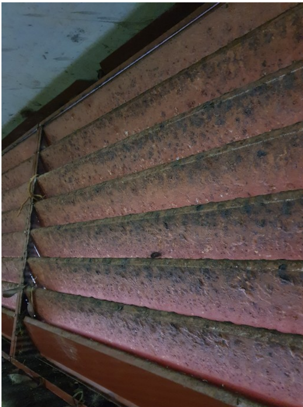
44 Louvres in basement repainted in 2018 and its status shown as of October 2021
