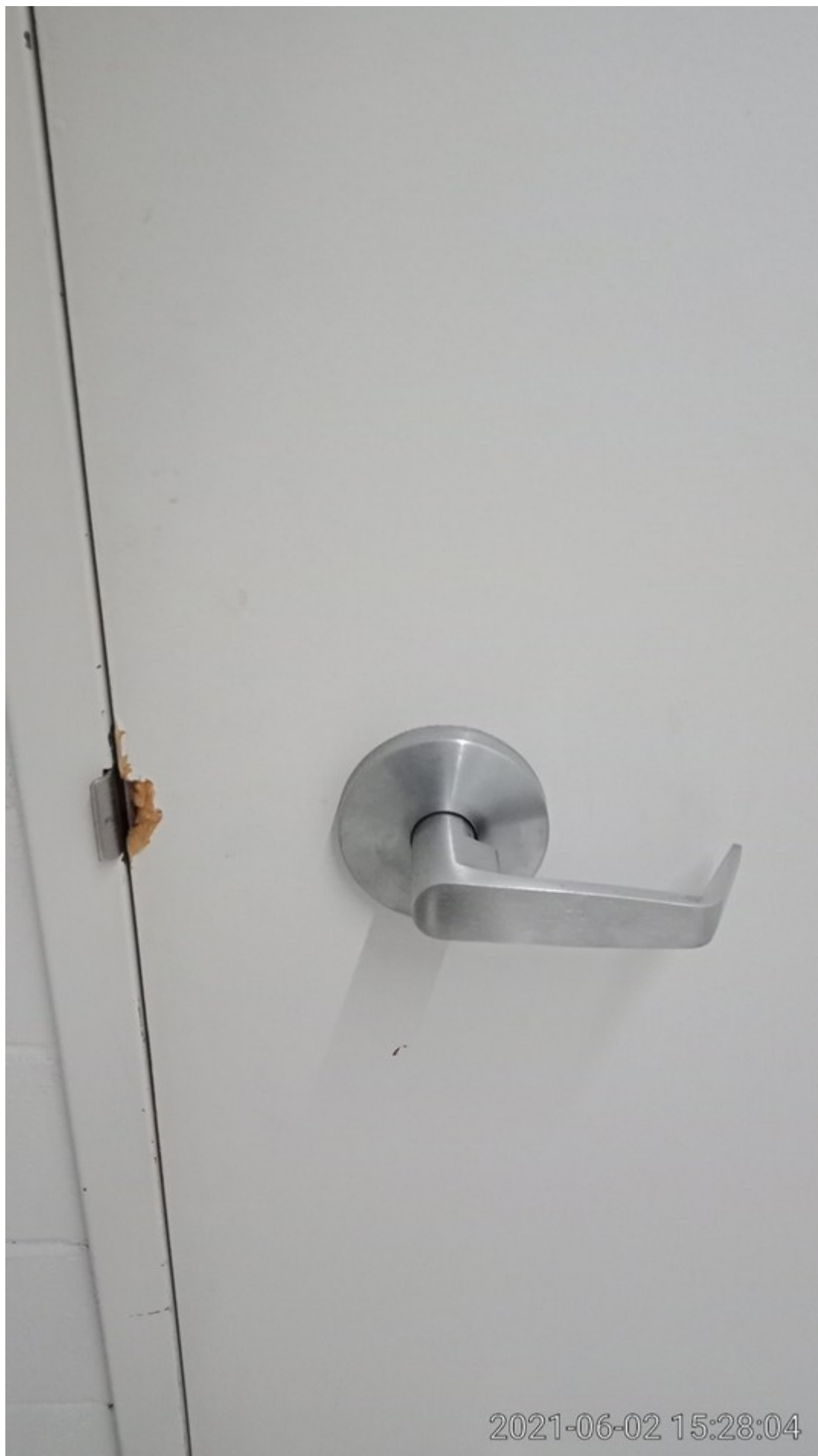
23 Damaged lock mechanism on fire door for two years – Block C ground floor
