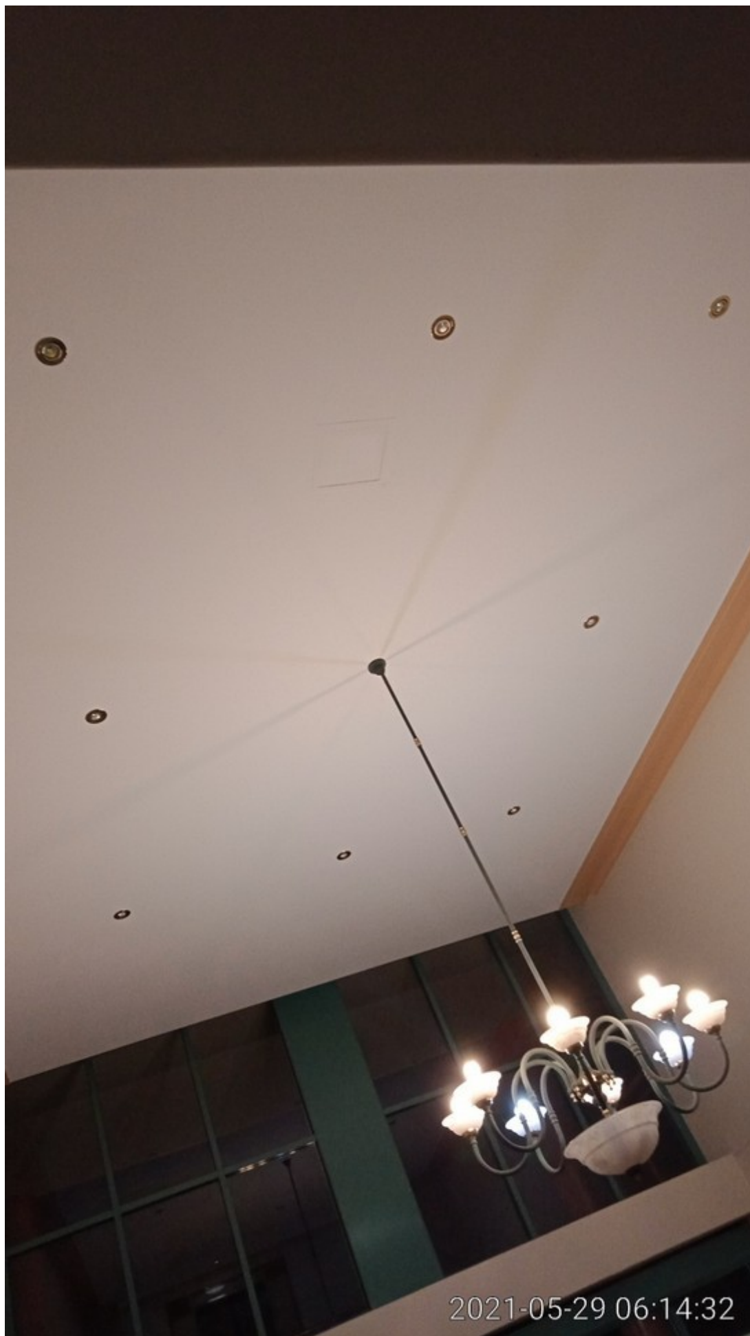
c) Block C, none of eight down-lights operational
