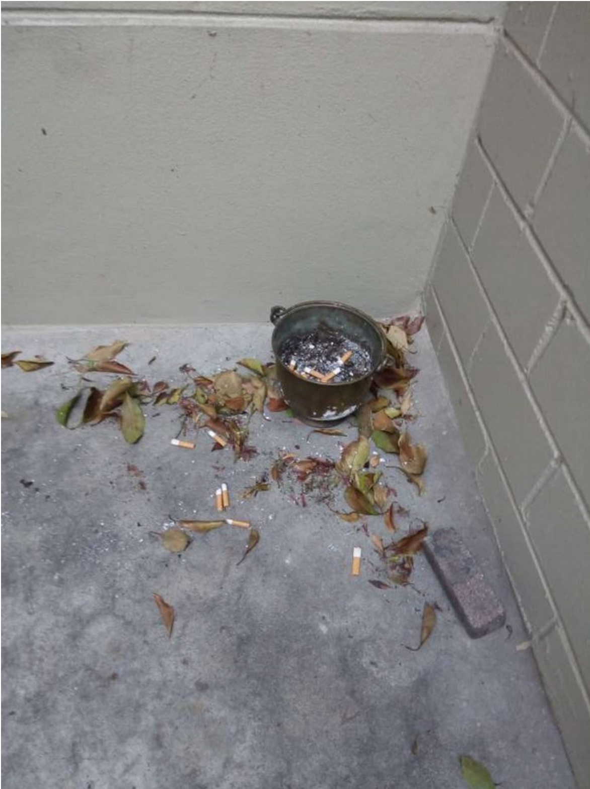
Example of smoking near fire door 2 below Block A in November 2018:
