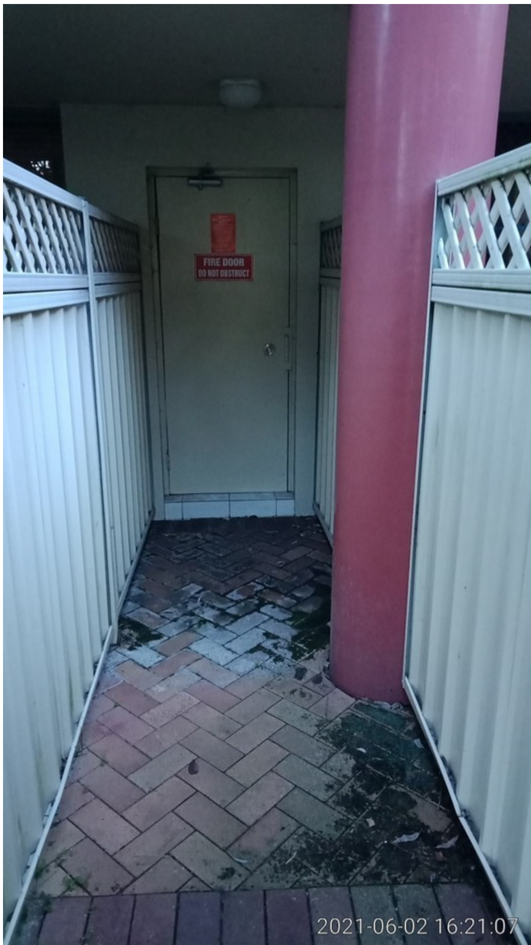
24 Appearance of pathway outside Block C fire door – slippery and mouldy for 14 months
