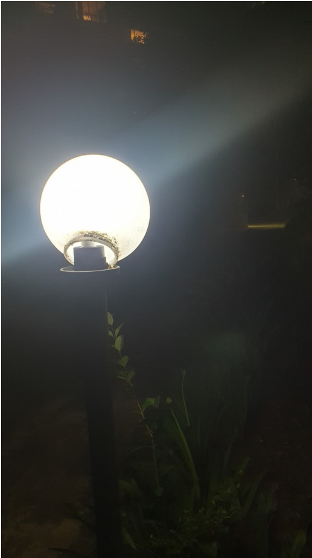
SP52948 – damaged light post globe behind Block D on 19 th of October 2021
