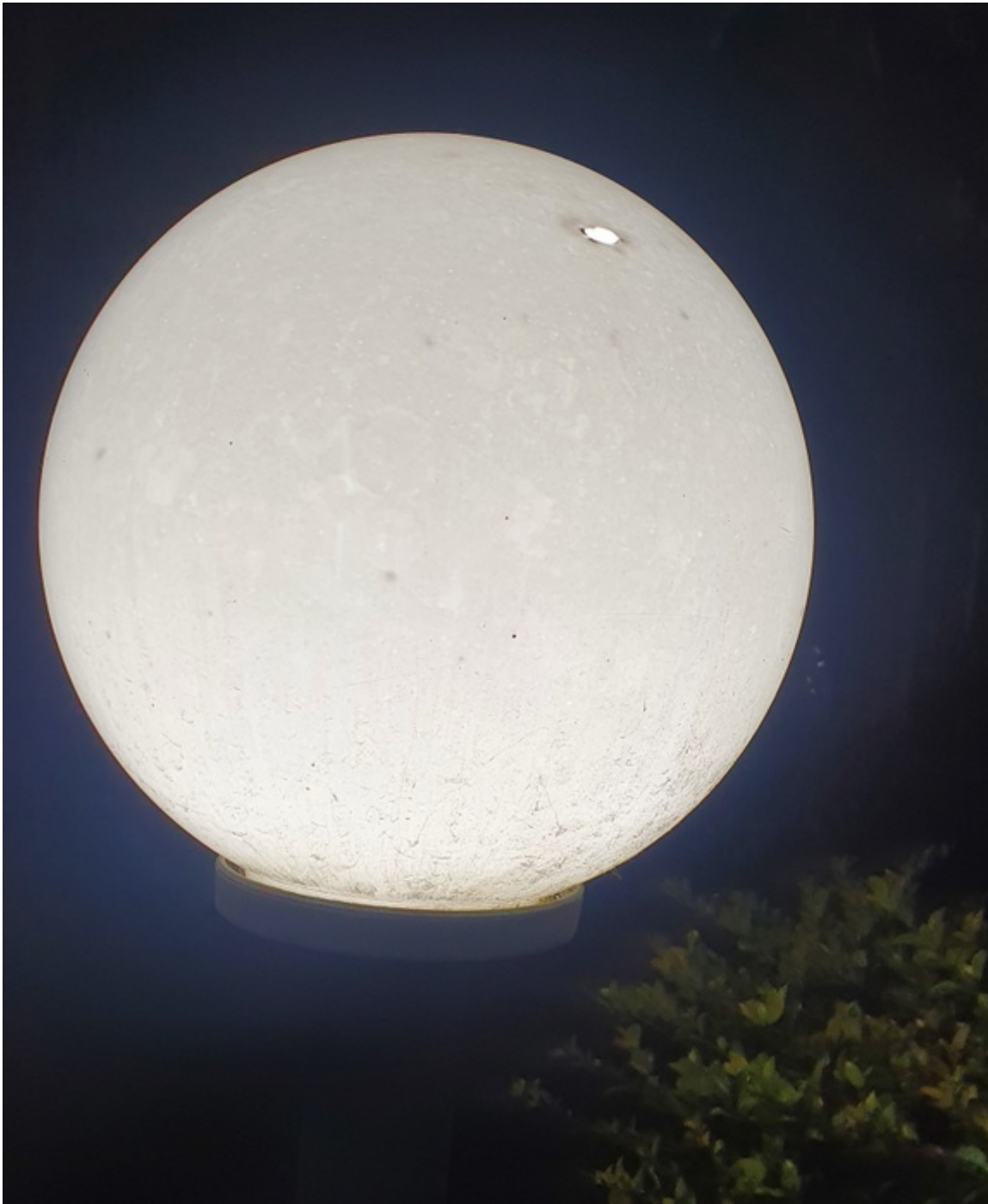
SP52948 – damaged light post globe near townhouse on 19 th of October 2021
