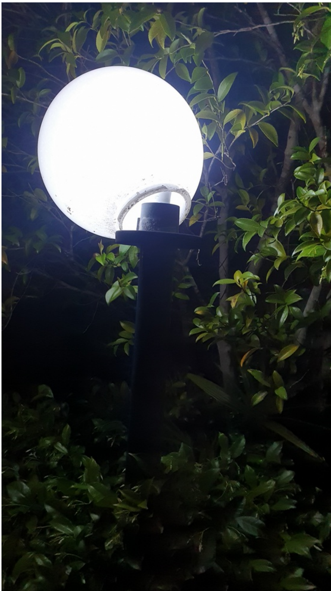
SP52948 – damaged light post globe near tennis courts on 19 th of October 2021
