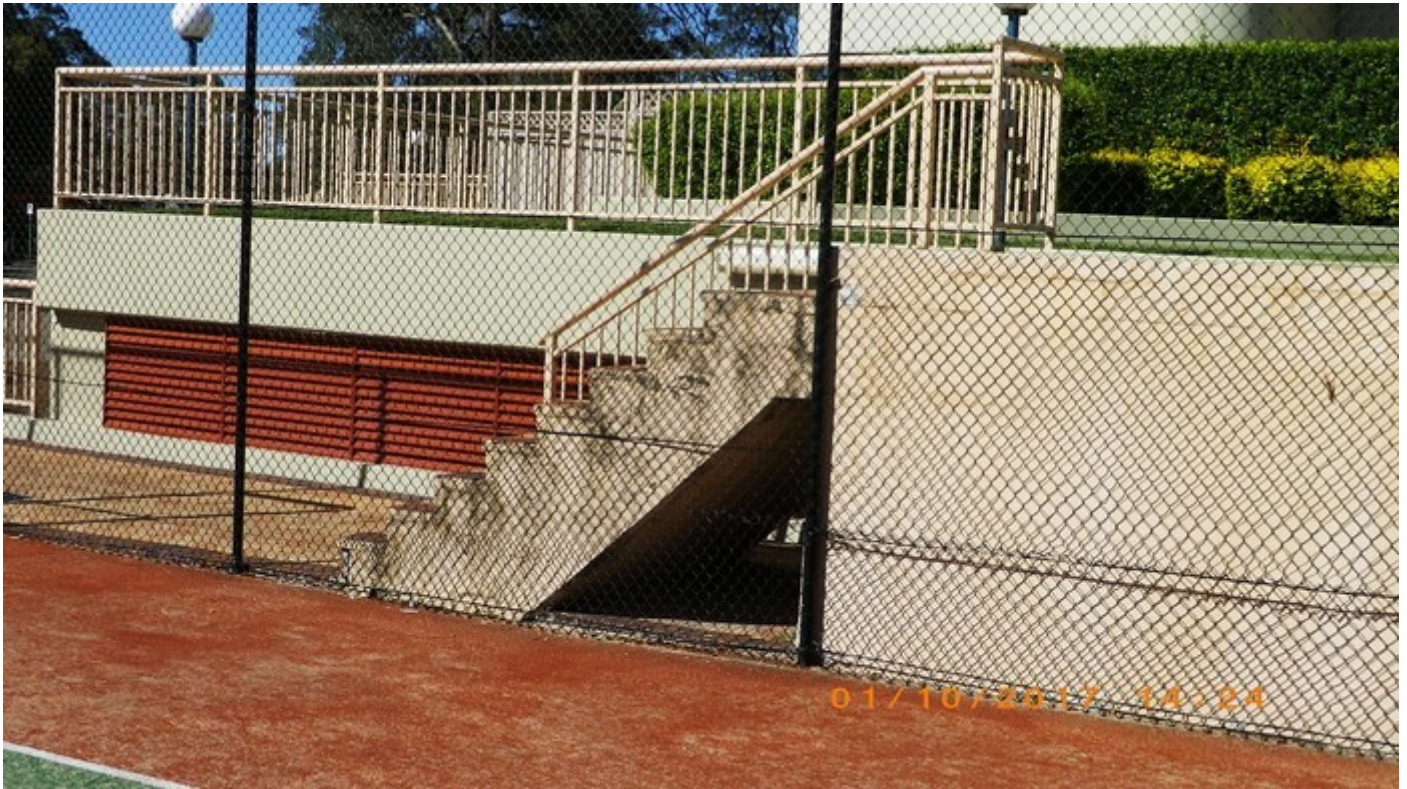
Building complex just repainted but not everything included in SP52948
