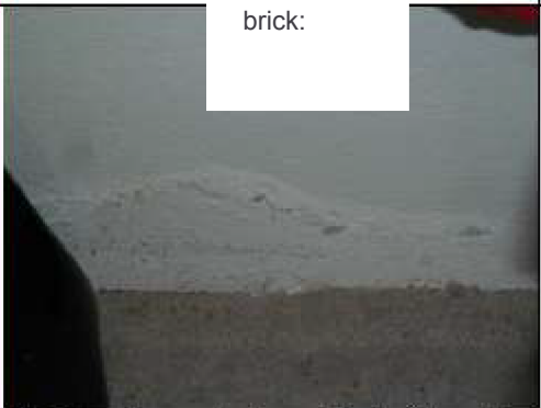
Moisture damage to base of walls internally of unit 151
