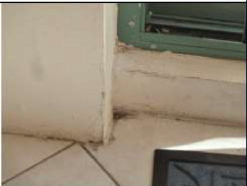
Moisture damage to hob wall of sunken patio area within unit 150
