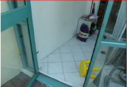
Area of sunken enclosed patio wall within unit 146 that requires installation of an air-stallatio-brick:
