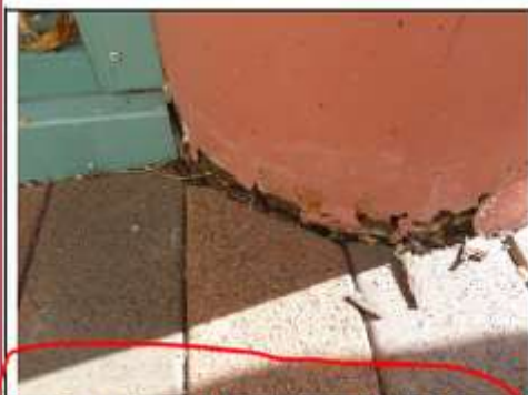
Concrete spalling at base of unit 150's enclosed patio area column
