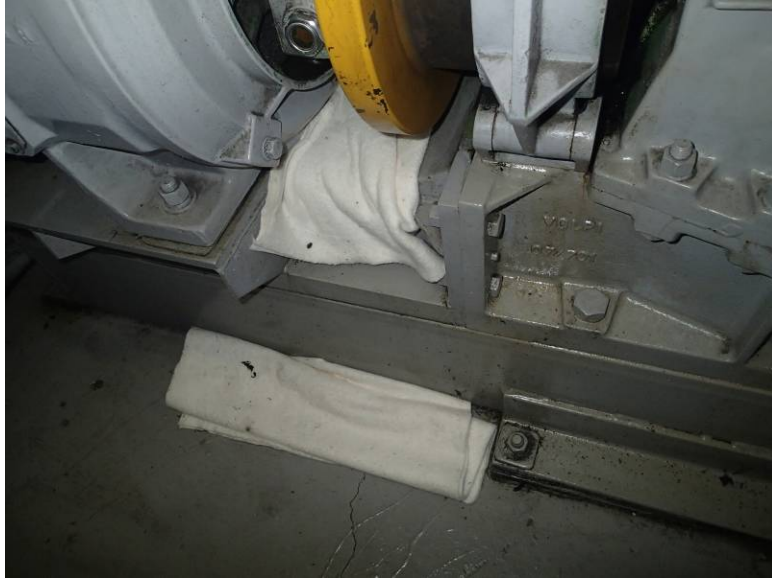
Hoisting machine oil leaks must be repaired and oily rags removed
