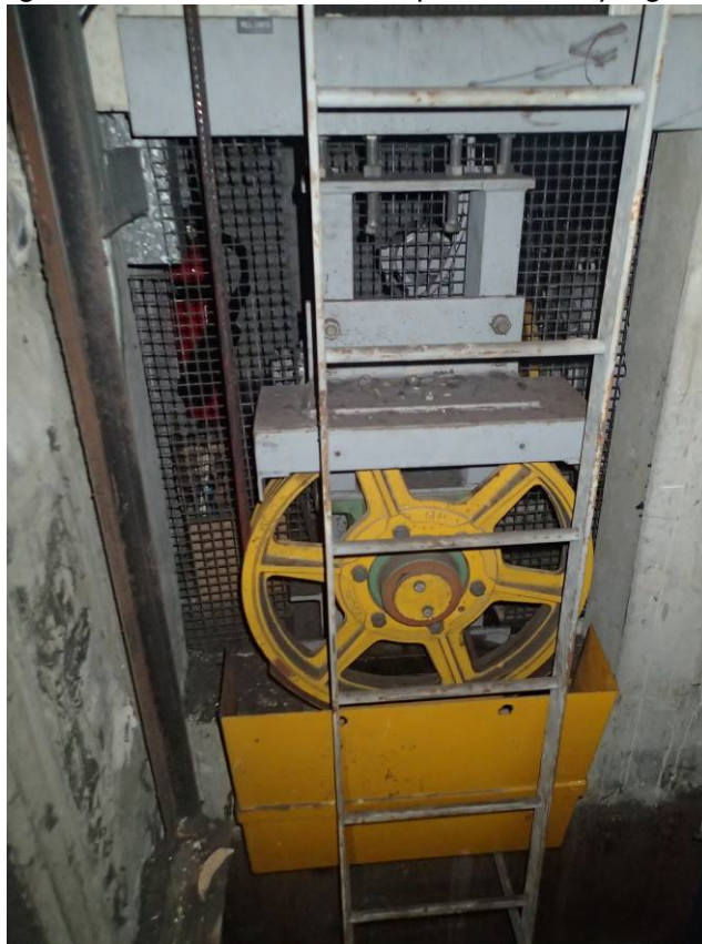
Traction sheave guards must be correctly installed
