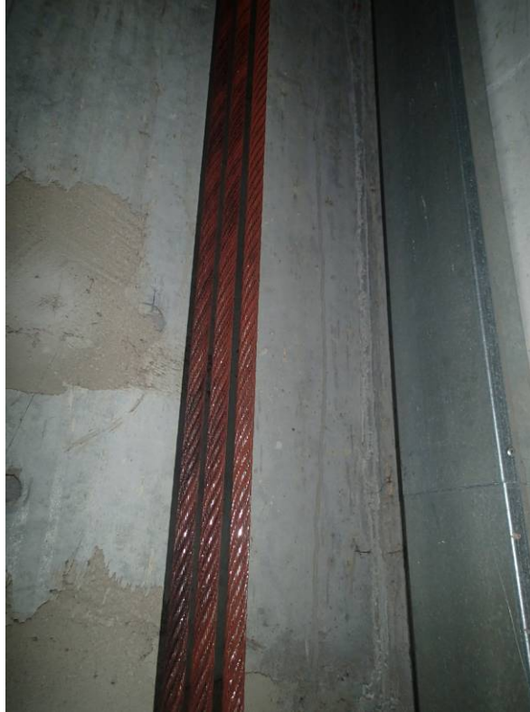
Rusty hoisting ropes must be replaced
