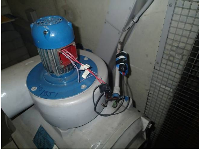
Hoisting machine fan wiring must be correctly terminated
